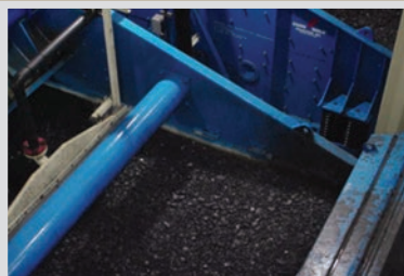
Coal handling and processing activities at Poplar Grove.
