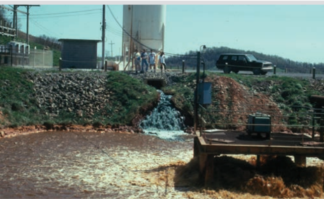
Typical Acid mine drainage (AMD) treatment plant: Lime addition, aeration
